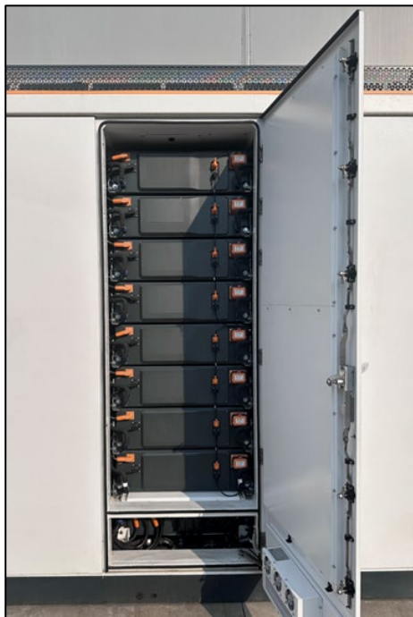
Figure 3: Battery Rack (Total 10 Racks for BESS Container)
